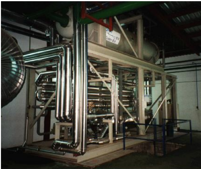
Figure 5 The ARP installed in a vegetable freezing factory in Talavera (Spain)
