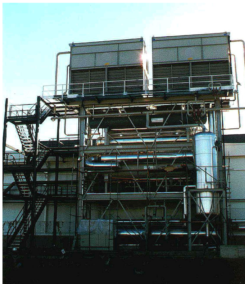
Figure 1 The ARP installed in a meat factory in Logroño (Spain)
