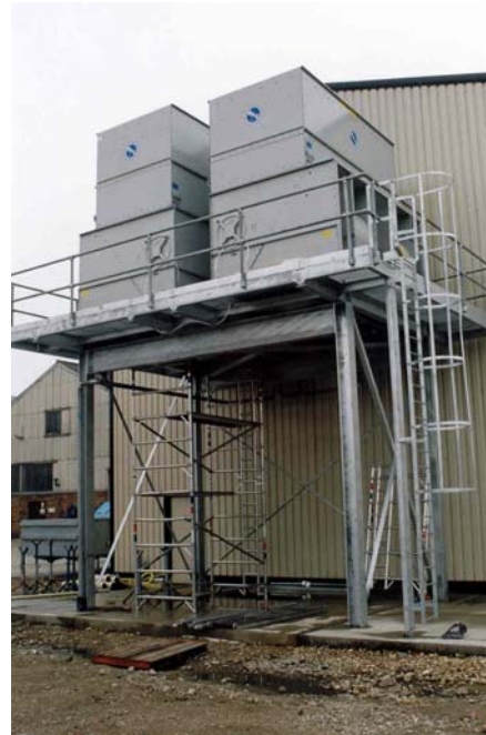
view of the two Baltimore evaporative coolers
