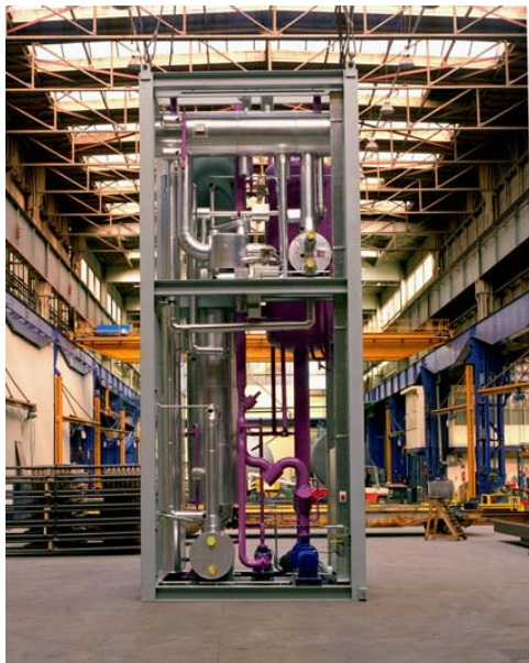
view of the indoors part of the installation
